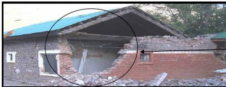
Stage III of Earthquake. Damage
