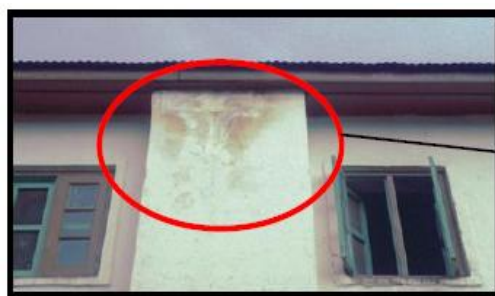
Stage I of Earthquake. Damage
