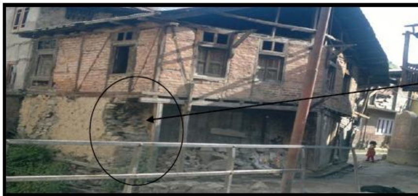
Stage III of Earthquake. Damage
