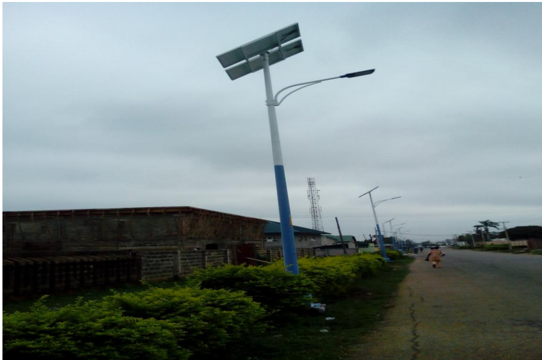
Figure 2: solar street lights with wrongly placed battery
