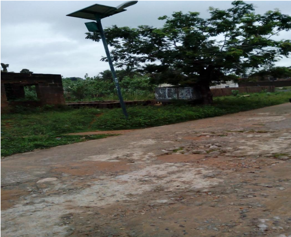
Figure 1: A solar street light installed very close to a tree.
