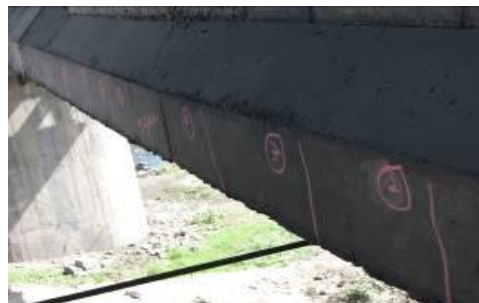
Figure 2: Cracks in main beam
