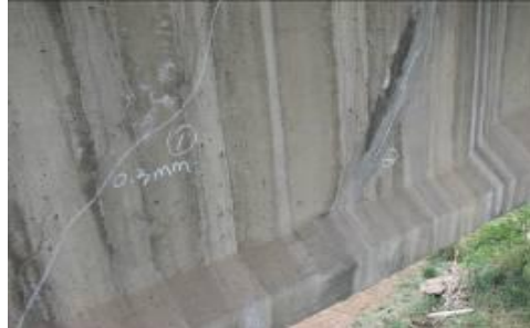
Figure 1: Diagonal shear cracks on web near supporting seat
