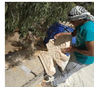
Image ( 34 ) shows The beginning of placing and installing one of the sharrafat
