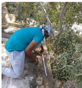
Image ( 31 ) shows Taking measurements of the missing areas of artificial stone formations(sharrafat)
