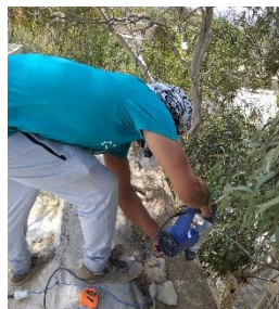
Image ( 32 ) shows Perforating the places of the coils to install the artificial stone (sharrafat)
