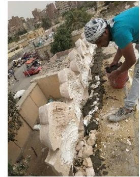
Image (37 ) shows Apply cement mortar to the linen ties and galvanized mesh attached to the coils Place the broken pieces with mortar from the damaged sharrafat
