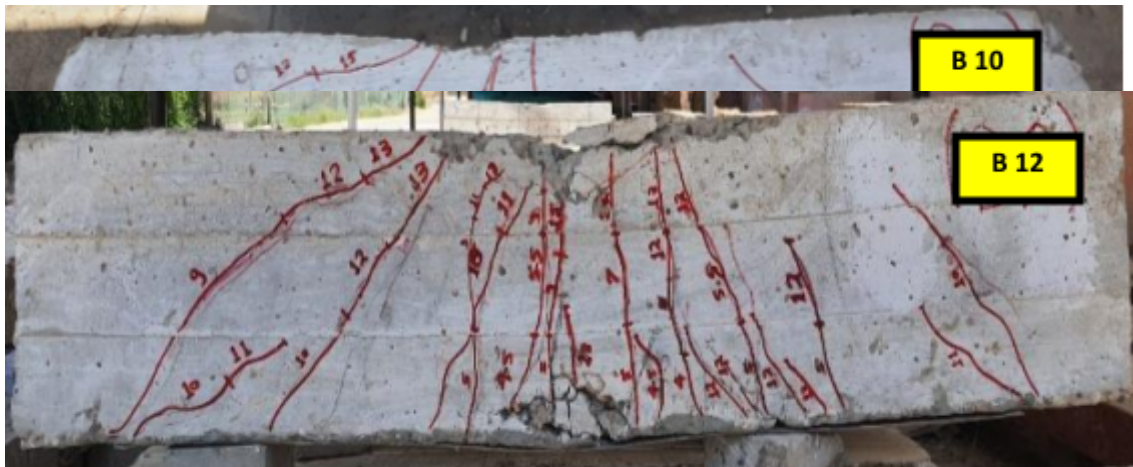
Figure 8: Failure Mode and Pattern of cracks for strengthened beams at group (II)
