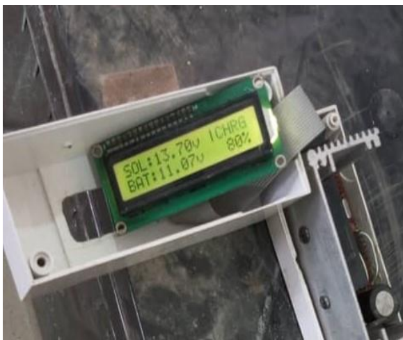
Figure 4: when the battery voltage is below the rated voltage the charge controller charge the battery via solar PV
