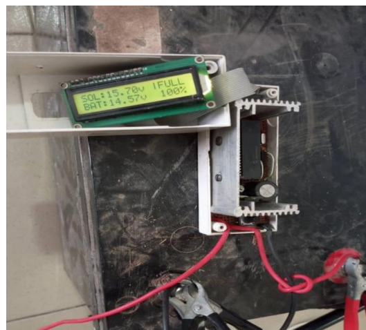
Figure 5: when the battery is fully charge via solar PV
