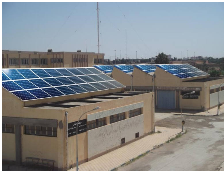
Figure (8) The default format for the installation of matrimonial plates on buildings.
