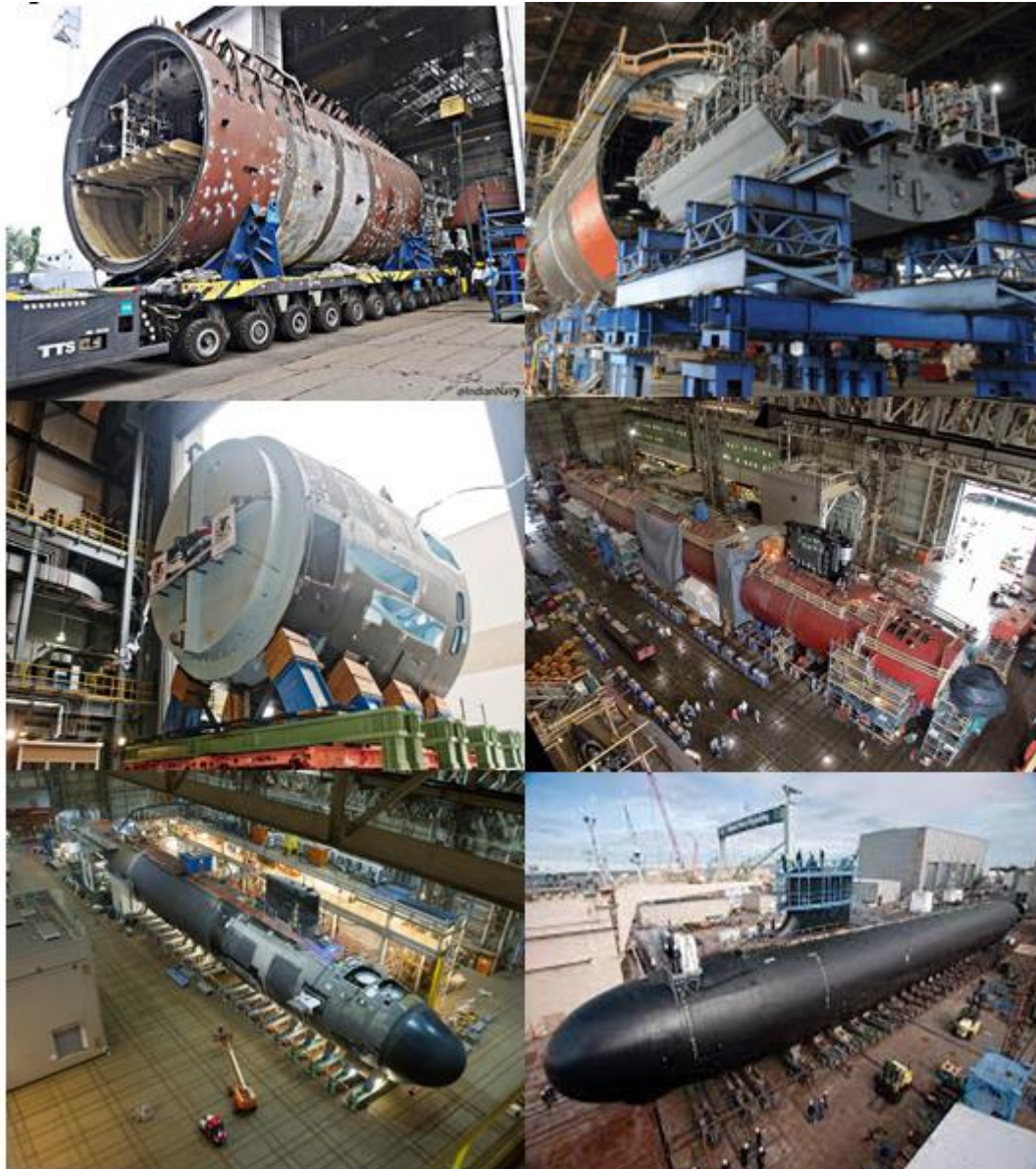
Figure 13: Modular Construction of Submarine (Virginia-class Nuclear Power submarine of the US Navy) 37
