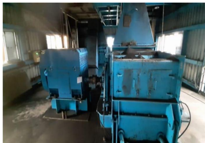
Fig. 4. Coal crusher unit on the coal handling system.
