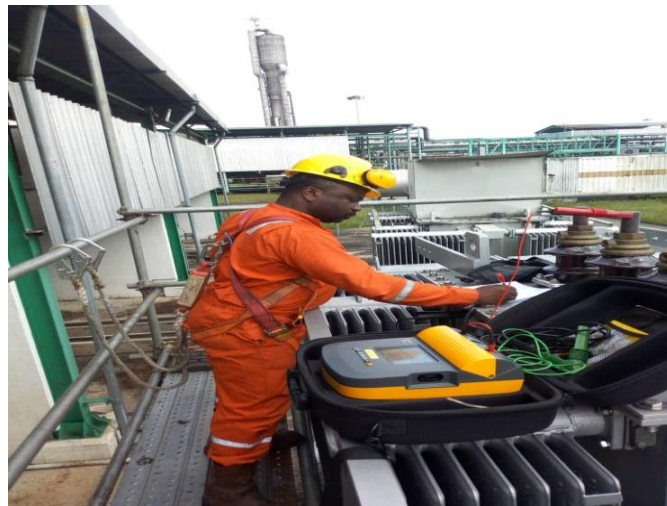
Figure 1: Megger test on 11KV 30MVA reactor in Nigeria Agip Oil Company, Obrikom.
