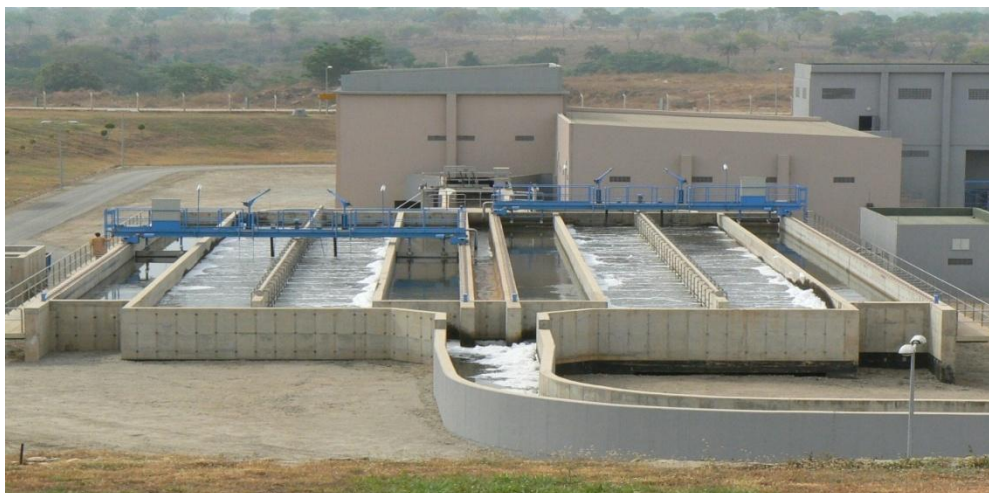
Figure 2.2: Shows first part of Wupa Wastewater Treatment Plant
