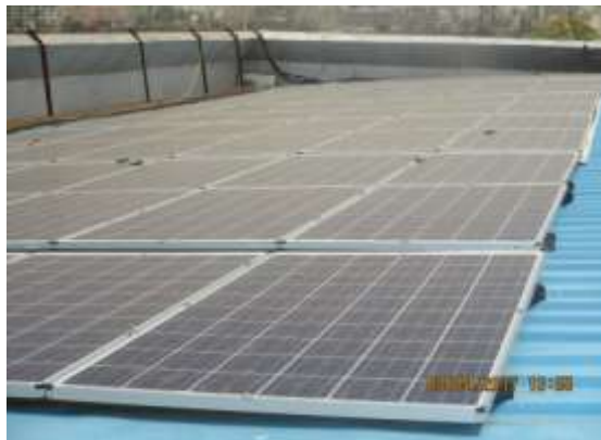
Figure 1: 15 kW Roof-top solar PV system at ECN, Abuja.
