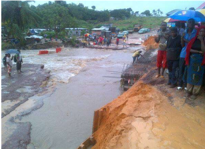
Fig.1: Road in a state of disrepair and carried away by rain in Brazzaville
