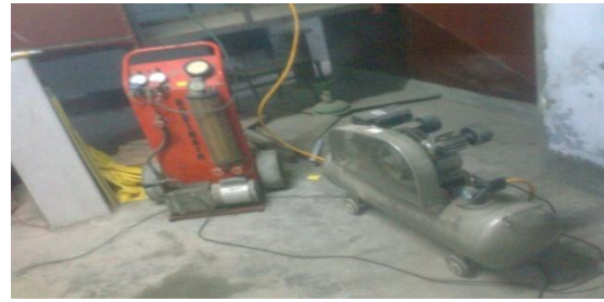
Snapshot of high pressure compressor and low pressure vacuum pump
