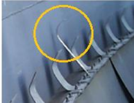
Figure 3: Shunt Not Making Contact with the Tank Copyright: Lightning Eliminators and Consultants, Inc. 2012
