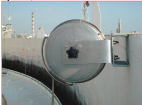
Figure 4: Retractable Grounding Assembly Copyright: Lightning Eliminators and Consultants, Inc. 2012
