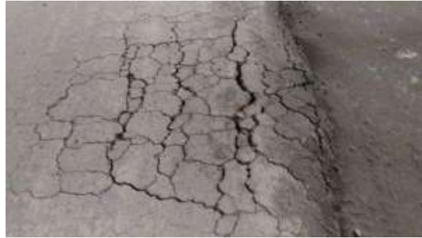
Figure 1. Example of asphalt damage after being passed by vehicles because of wet BCA before pavement.
