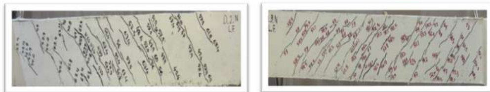
FIG.8. Side view of beam D2N at failure Fig.9. Side view of beam D3N at failure
