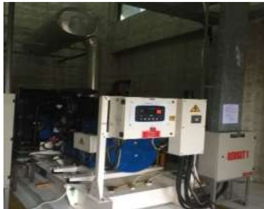
Fig 1. Unit Diesel Power Plant 220 kVA
