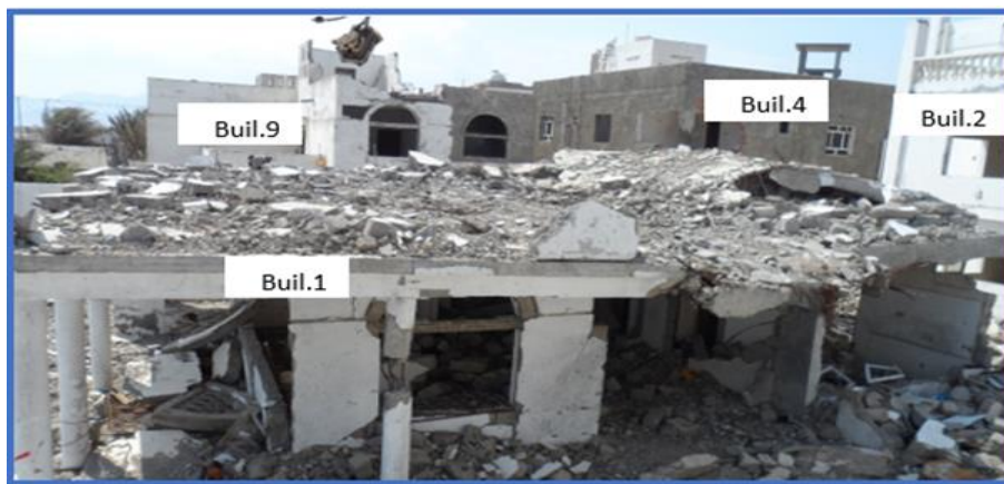
Figure 26: Damages in buildings 1 & 2 that directly exposed to bombing and in buildings 4 & 9 that indirectly exposed to bombing
