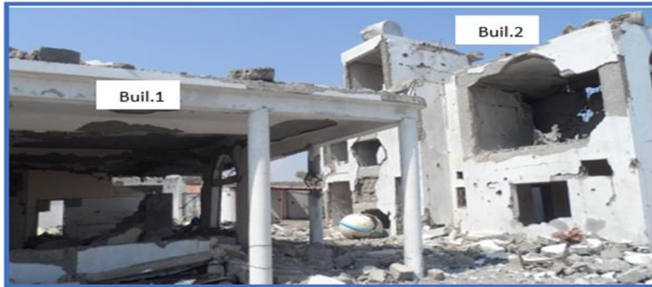
Figure 25: Damages in buildings 1 & 2 that directly exposed to bombing
