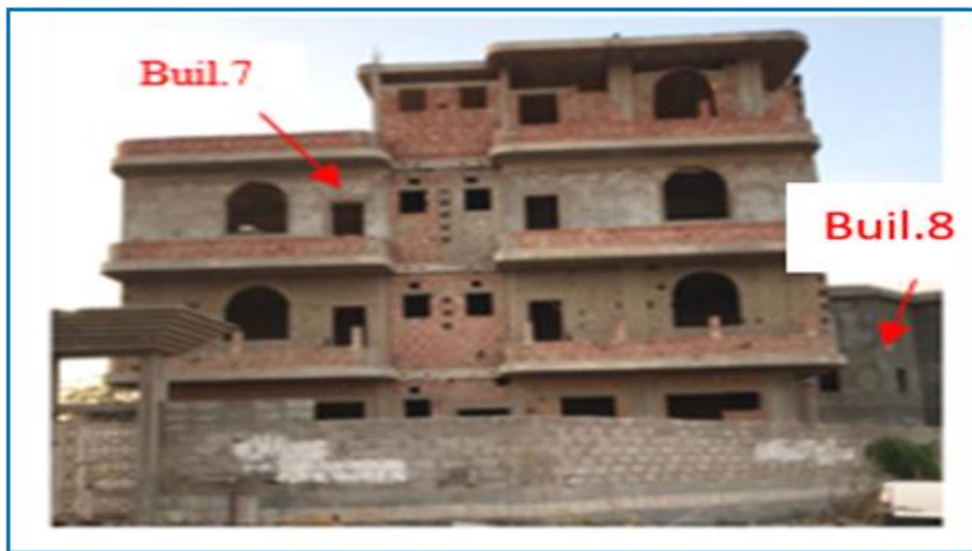
Figure 29: Damages in building 7 & 8 that indirectly exposed to bombing
