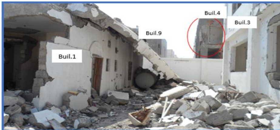
Figure 27: Damages in building 1 that directly exposed to bombing and in buildings 3, 4 & 9 that indirectly exposed to bombing
