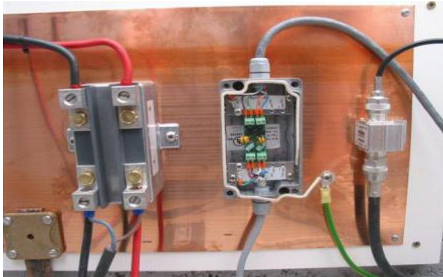
Plate 2: Examples of practical design and installation of equipotential bonding bars
